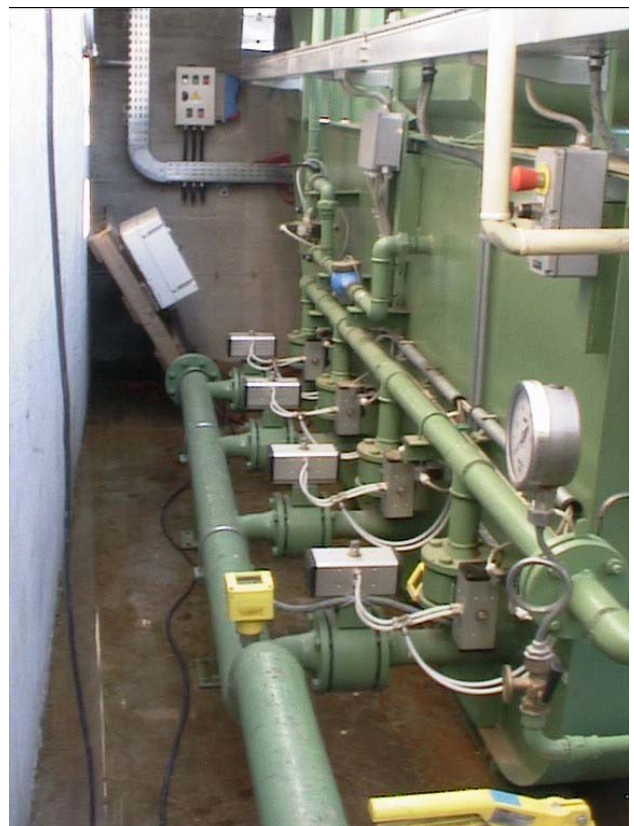
Suction and back wash pipe.
